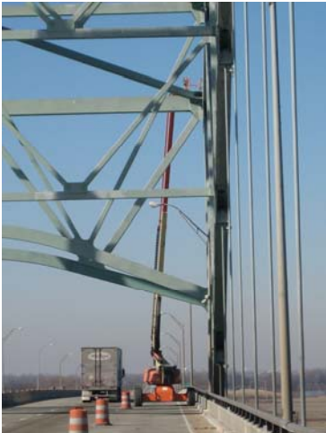
Two team members are lifted to the lowest point of the bridge truss.
