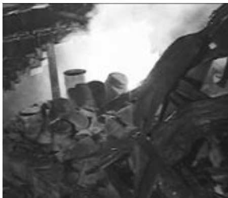
The wireless Pan/Tilt/Zoom Construction Camera, which enables us to preview the dangers in a worksite before entering, captures a magnesium/lithium flare-up at a job site in Arkansas.
